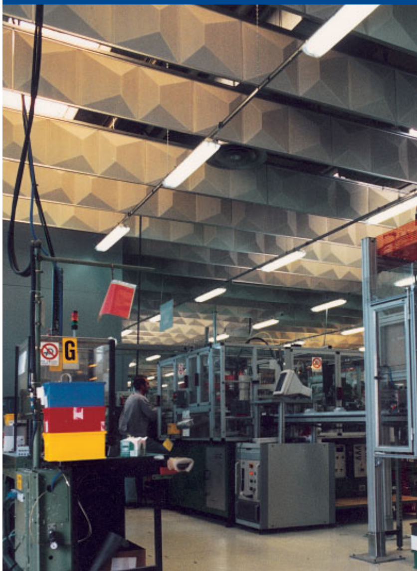
2 Valphon 400S sospeso a baffles in ambiente industriale. VALPHON 400S SUSPENDED IN BAFFLES IN AN INDUSTRIAL ENVIRONMENT.
